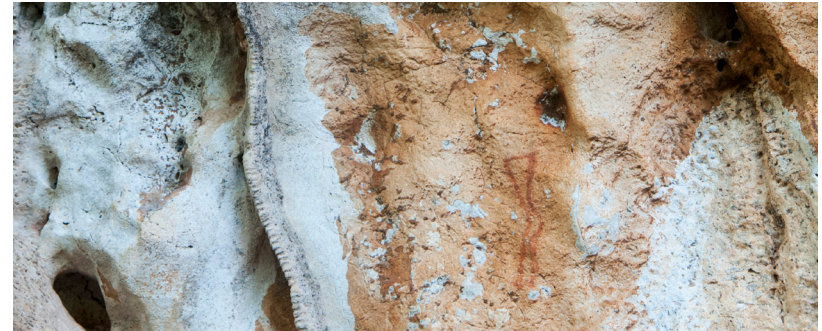
Figure 7: The compact ochre weathering crust as support of pictograms tends to detach and finally falls off (Momi Momi Raka). (Photograph taken by Prof. Hans Leisen)
